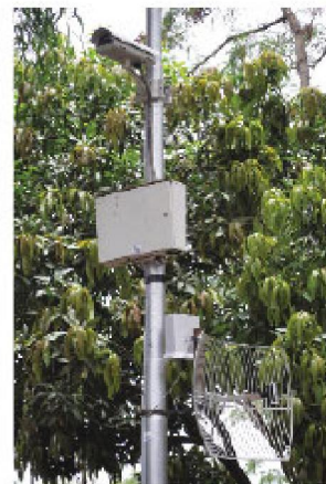
Surveillance Camera at MPA Nashik monitoring the perimeter on Milestone XProtect Corporate Open Platform Video Management Software
